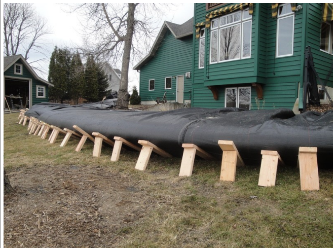
Many 2-board braces are in place along the side of the partially filled AquaDam.
