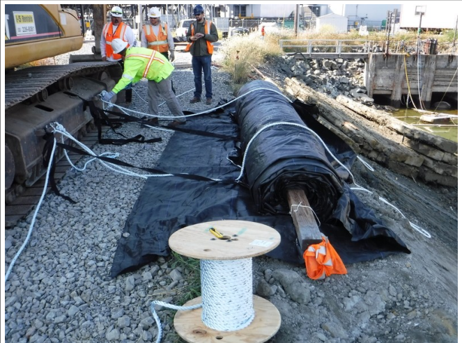
8ft tall, 100ft long AquaDam sits at the top of the starting bank
