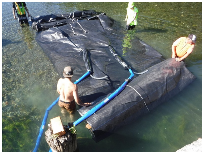
Two blue-color hoses are used to fill the two AquaDam inner tubes
