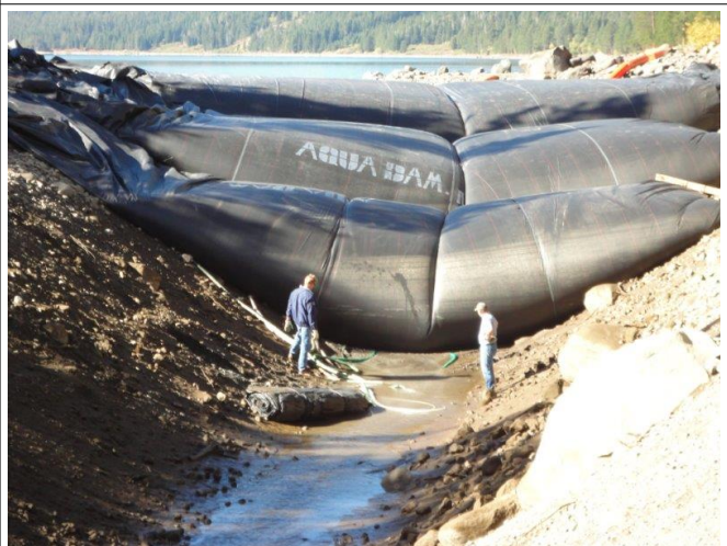
6ft tall men, 10ft, 16ft, and 21ft tall AquaDam (foreground to background)
